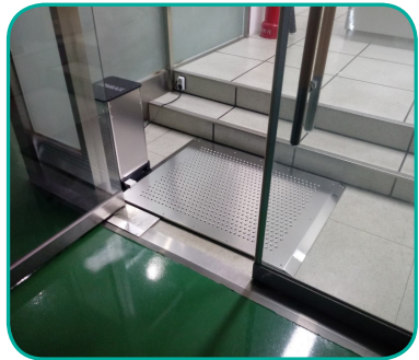
Product installed in KHNP, Hangang Hydro Power Site's Dcs Room
