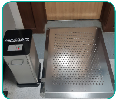
Product installed at the entrance of Control Computer Room of Busan Power Plant
