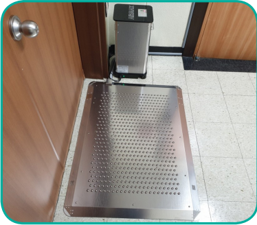
Product installed in Power Plant of Seoincheon
