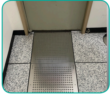
Access Type installed in Central Control Office of Bundang Power Plant
