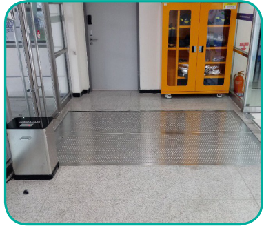
Embedded Type installed in Sinboryeong Thermoelectric power Plant
