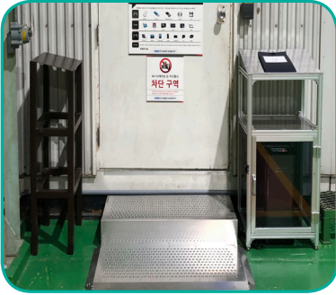
Stairs Type installed in 1 block B of Bundang Power Plant
