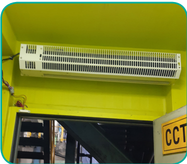
Air Curtain installed in Donghae Thermal Power Generation Department
