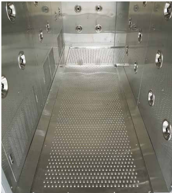
AIR SHOWER ROOM
