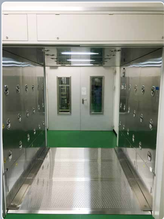
AIR SHOWER ROOM
